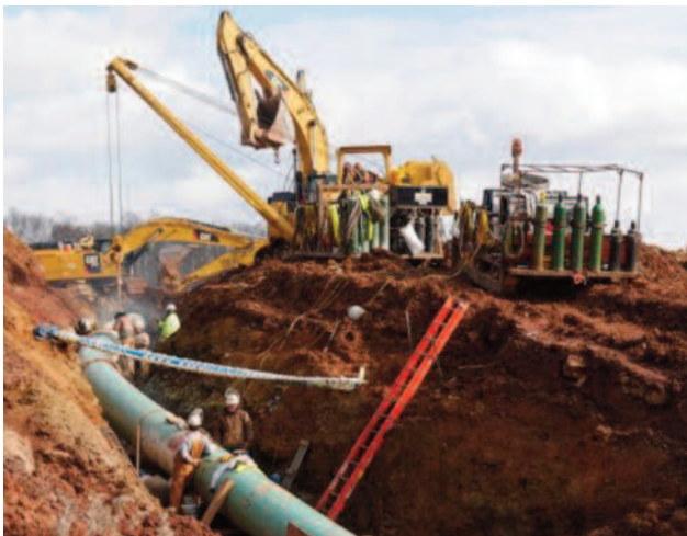
Construction of Blackstone's 713-mile Rover Pipeline, with Energy Transfer Partners, which is planned to cross through four states, Photo: Ohio Valley Environmental Coalition Dec. 2017
