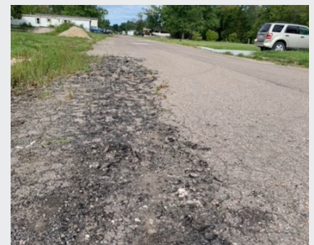
A broken road near Theo Gantos' home.
